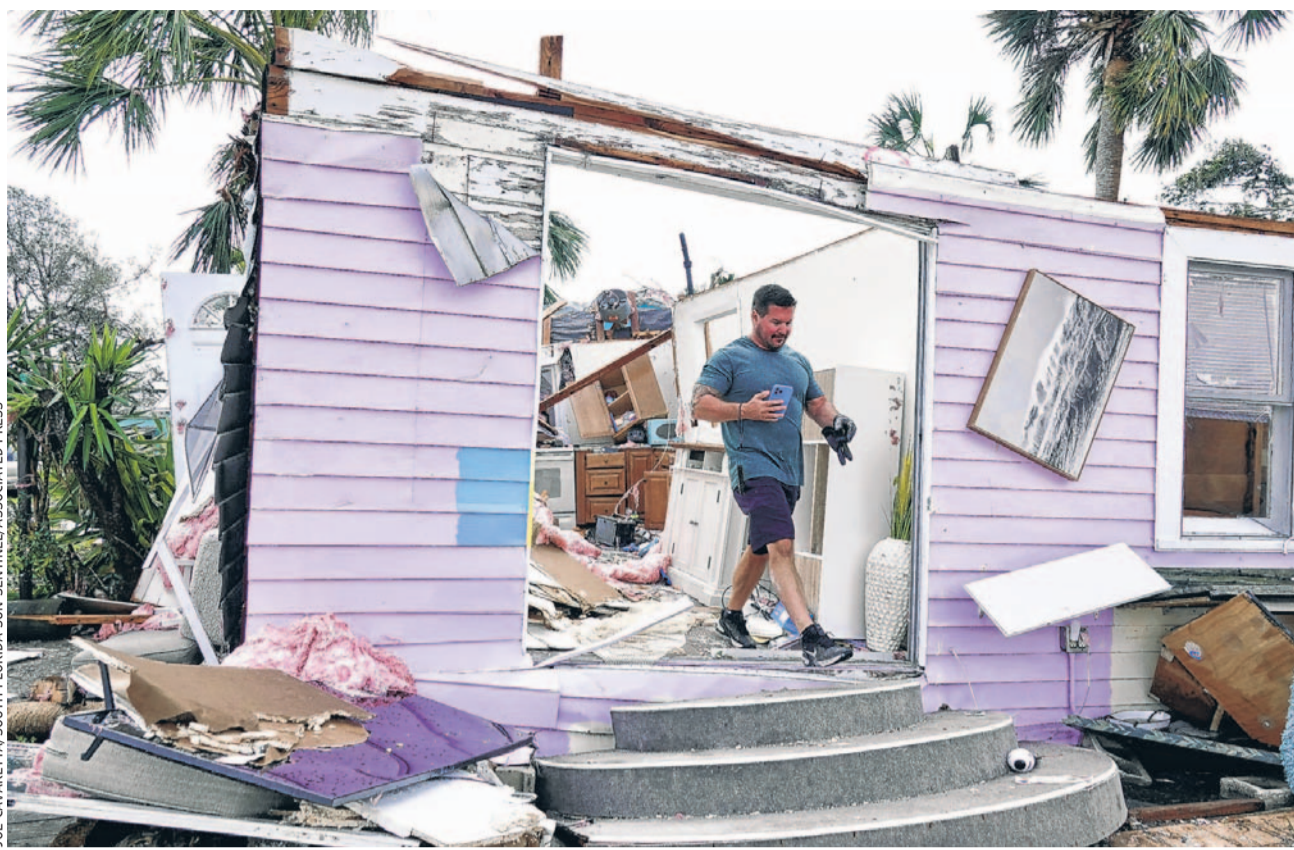
SMASHED: A man surveys the damage in Palm Beach Gardens on Sunday, the day after a twister crushed homes and overturned cars.
